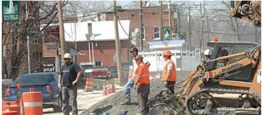
Construction crews tear up Main Street in Old Town St. Peters to make way for a new infrastructure. City officials are working on a plan that will enhance the downtown and will hopefully attract more businesses and residents.
